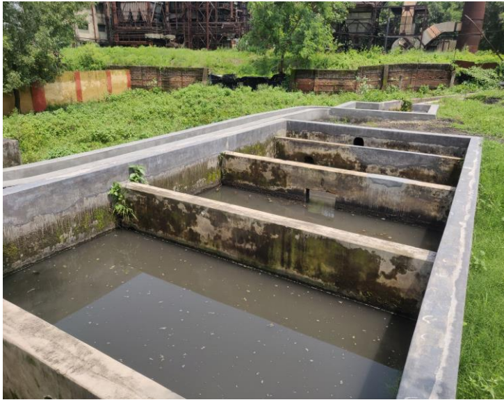
Oil & Grease Trap
